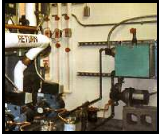
DAY TANK FAIRBANKS, ALASKA 1994
