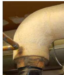
Boiler Supply Elbow
