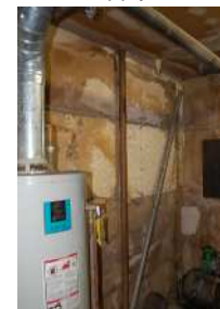
Water Damaged Sheetrock
