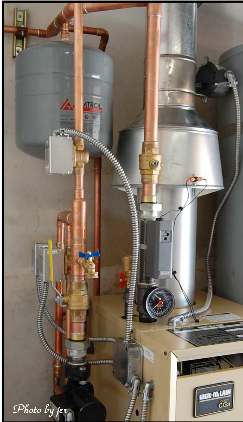
BOILER INSTALLED BY JERRY ANCHORAGE ALASKA (ACTUALLY VIEW OF PRESCRIPTIVE DRAWING)
